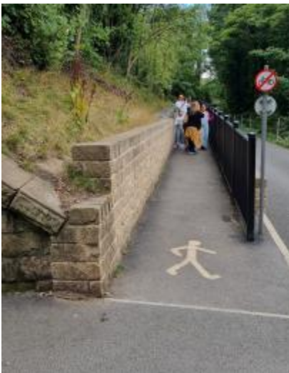
Photo shows the pedestrian route to the Heights, with a railing on the right to separate from the access road.
